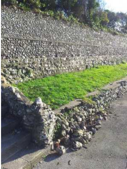
Flint walls around cycle track in state of disrepair
