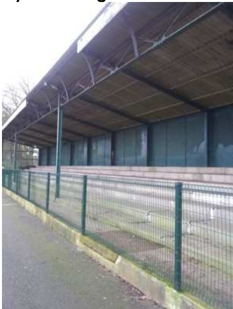
Cycle track grandstand in state of disrepair
