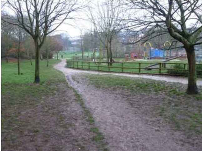
Footpath to playground eroded
